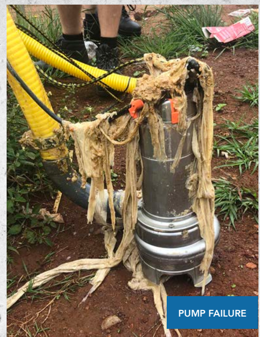
COMPLETE SYSTEM FAILURE
