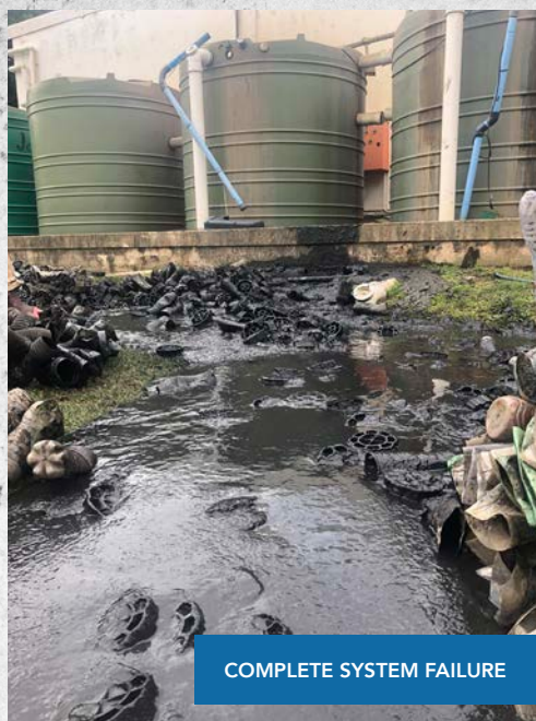
EXCESSIVE SLUDGE BUILD-UP
